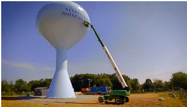
Photo: Final work being completed on a new Pennsylvania American Water tank in Canton Township, Washington County, in 2019.
